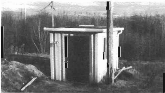
Station de pompage.
