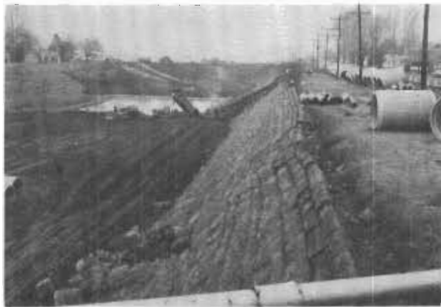
Filling in the new canal 1966-67. Showing the tile which are to go in at the bottom.
