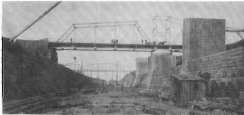
The new canal almost completed, the installation of the new bridge with the bridge that had been across the canal from Victoria Street.
