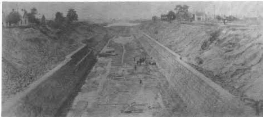
The building of the new canal at the Western end of the village.
