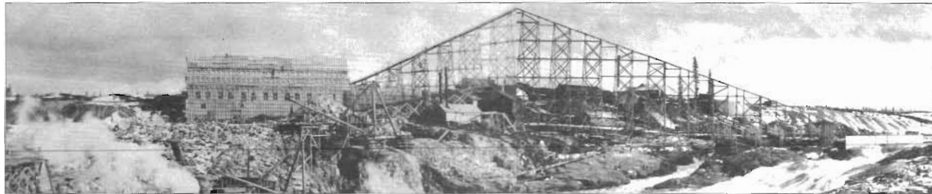
1916: The Mattagami Pulp & Paper Mill under construction / Construction de l'usine de la Mattagami Pulp & Paper
