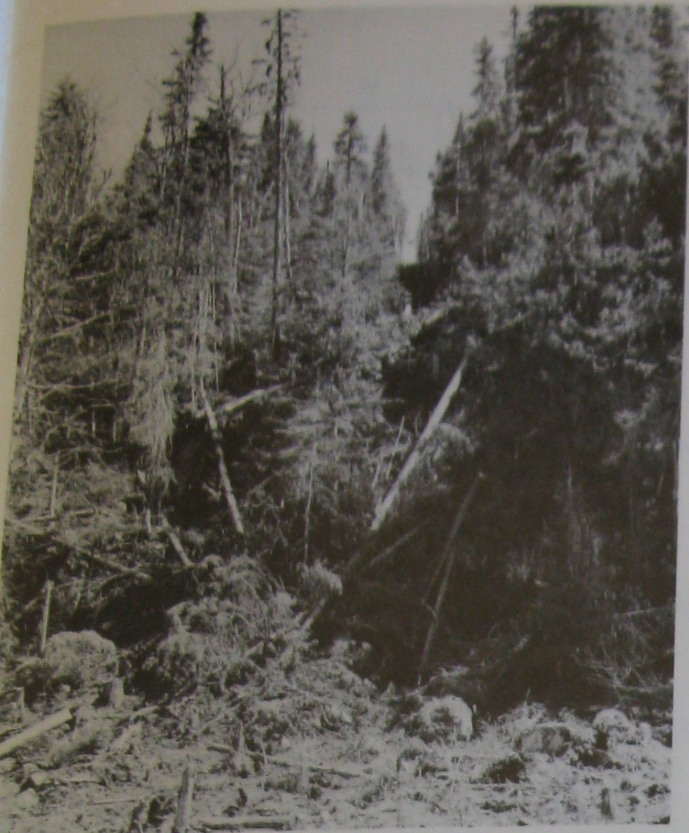
A broad swath through heavy timber was cut to make way for the Ontario Hydro line to the Geco mine.
